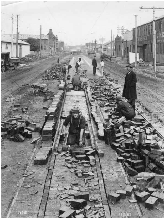
Woodblocking the new electric tram tracks. Can you pick the location? – Photo courtesy State Library of Victoria
